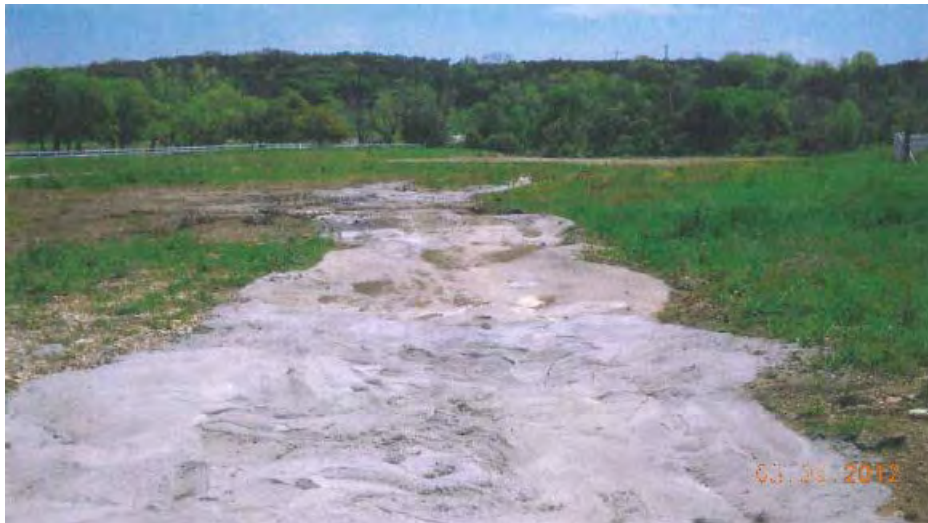
Repair of Erosion caused by Tropical Storm Hermine at Dam 4 Auxiliary Spillway
