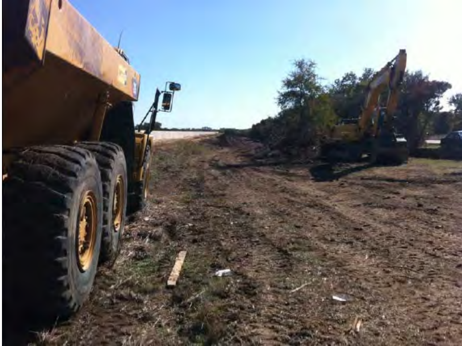
Repair of slope failure caused by Tropical Storm Hermine at Dam 13A
